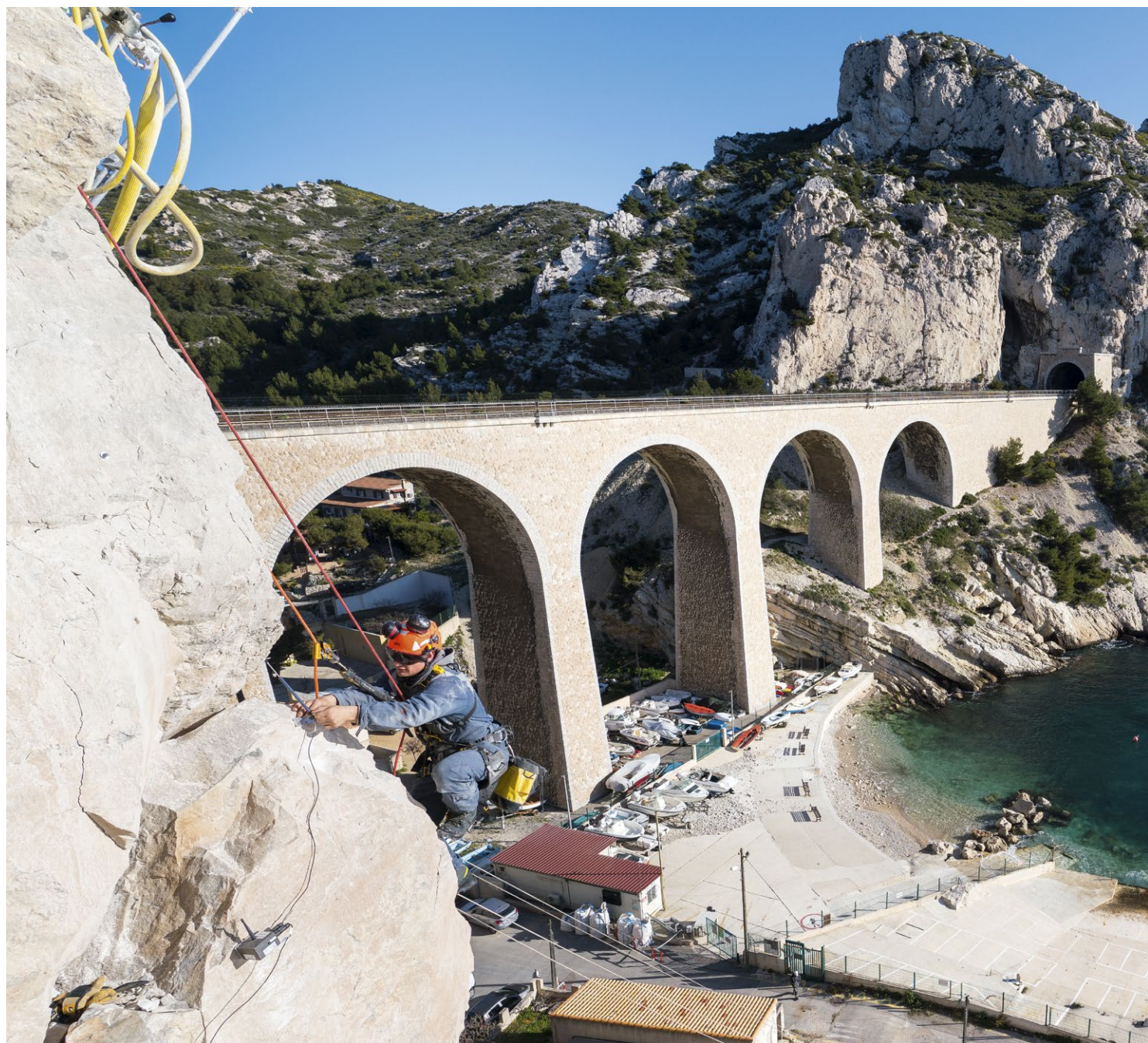
Rock fall protection works near Marseille, France. © 2020 Petzl Distribution - Vuedici.org - Profil - DDITM 13
